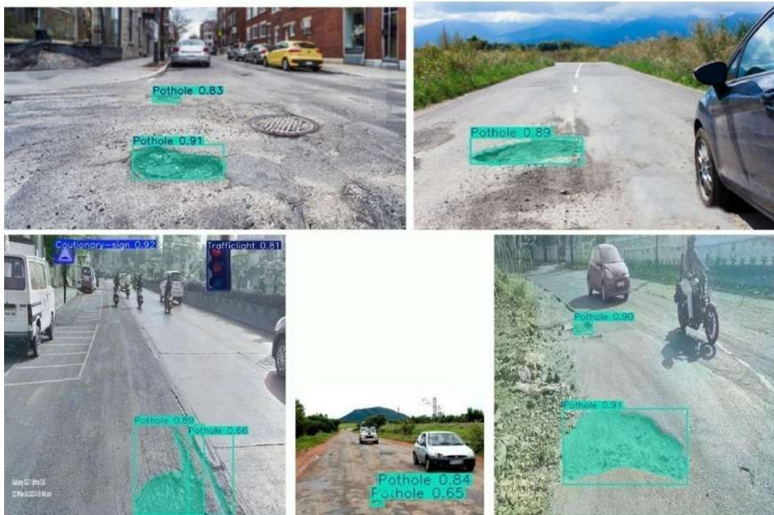
Figure 17: Predicting potholes in different conditions
